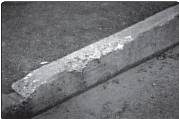
FIGURE 5: Concrete in the long run is susceptible to problems such as spalling.
