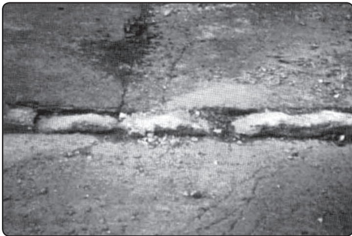
FIGURE 7: View of a completely deteriorated concrete curb.
