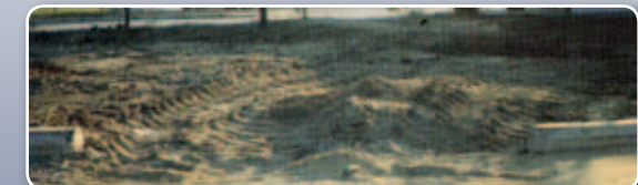
Here, a section of precast curb was completely pulverized by construction equipment at a shopping center.
