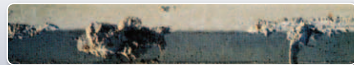
This precast curb was installed fifteen months ago and has been damaged by impact. It is highly susceptible to chemical freeze/thaw damage and will continue to disintegrate.
