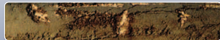
This eleven-month-old berm already is showing damage from compression and impact. Its useful life is almost over.
