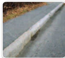
This granite curb was originally installed over 100 years ago in Milford, New Hampshire. It recently was re-installed due to road improvements and still looks great!
